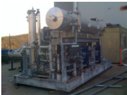
Figure 3A: Pre-combustion UNO rig before modifications.
