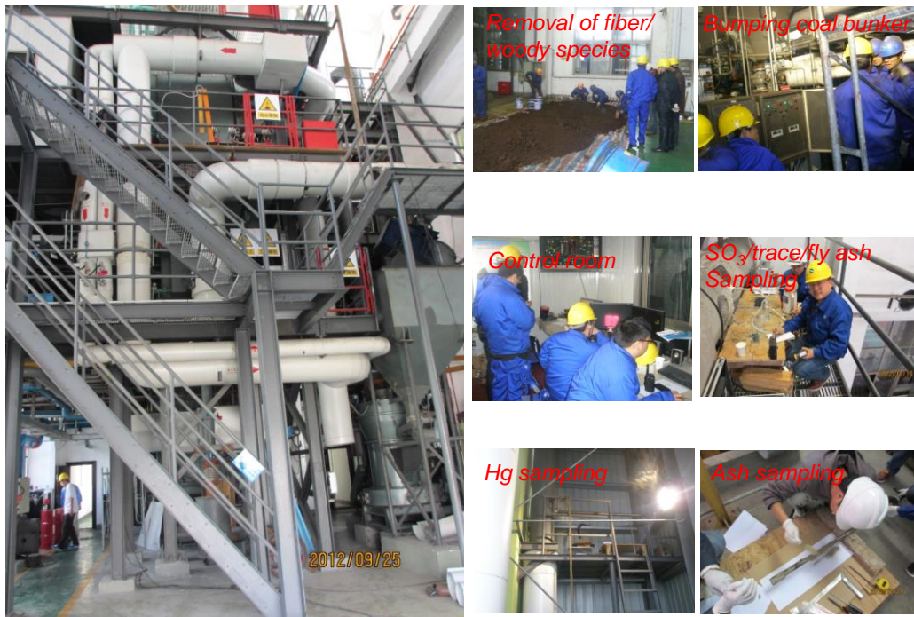
Figure 3.2 Front views of the SBWL 3 MWth oxy-firing facility and different units
