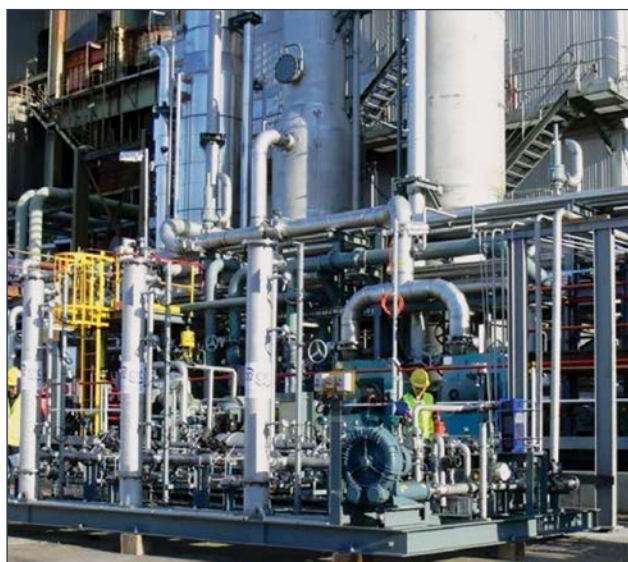
Figure 53: Pilot-scale adsorption rig at Hazelwood power station
