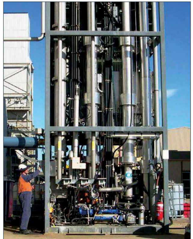
Figure 45: CSIRO post-combustion capture pilot plant at AGL Loy Yang power station
