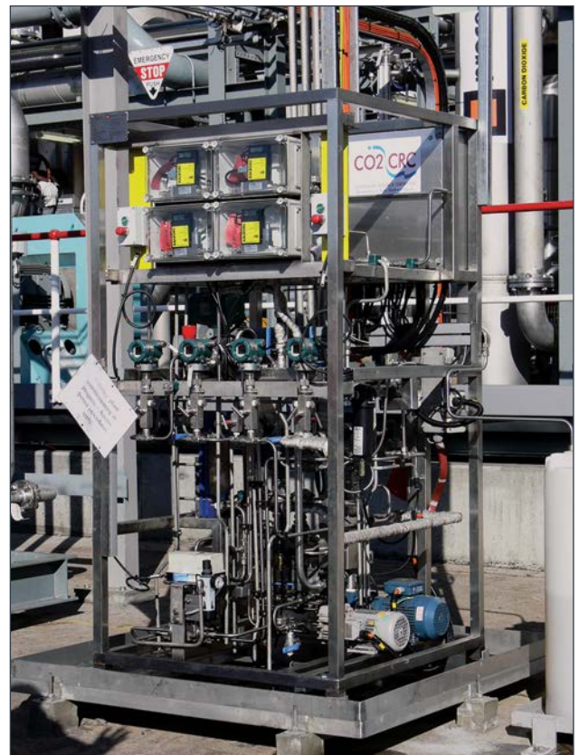
Figure 57: Membrane pilot plant at Hazelwood power station
