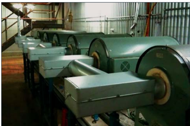
Figure 71: Steam oxidation facility at Loy Yang B power station
