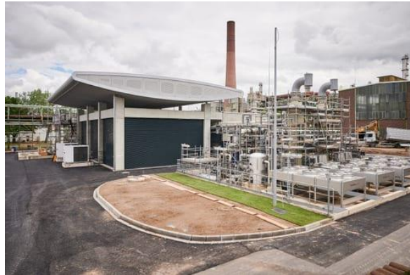
Figure 101: Europe’s largest PEM hydrogen electrolyser at Rheinland refinery 197
