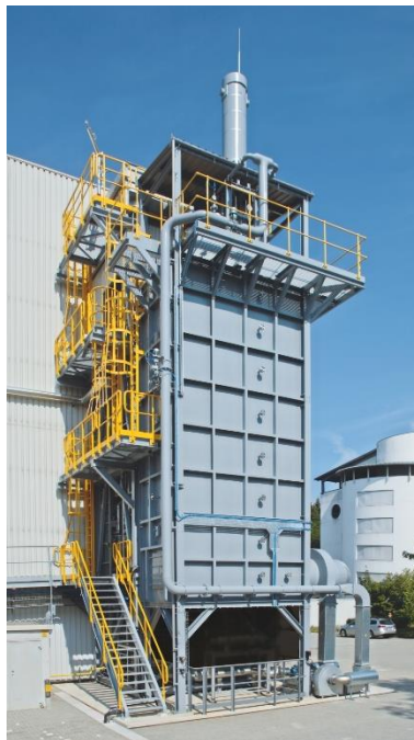
Figure 80: Linde Group dry reforming pilot plant 140
