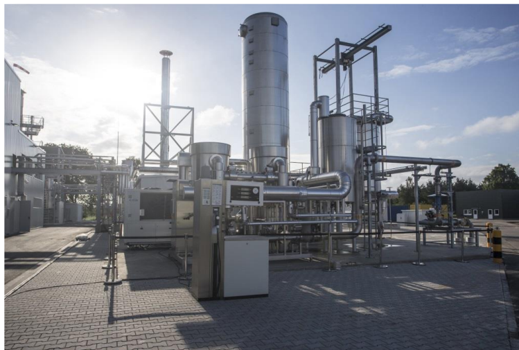
Figure 95: Audi e-Gas plant 187
