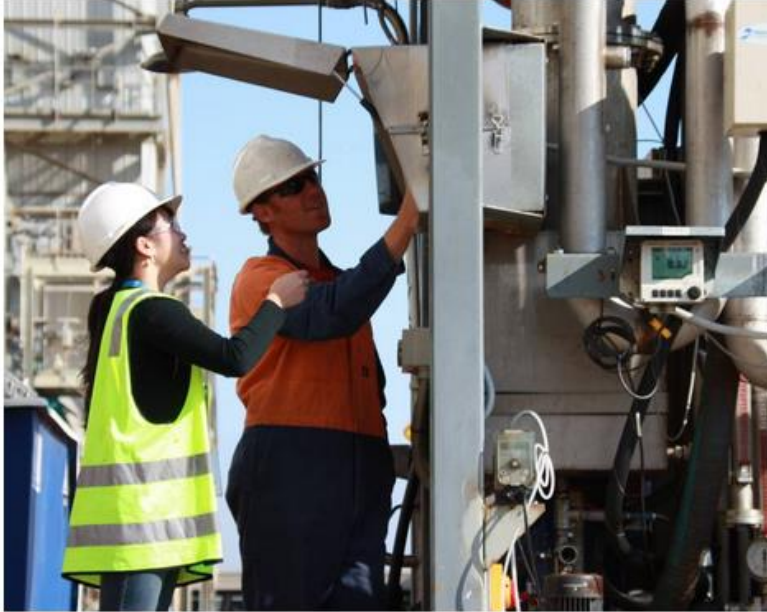
Above: CSIRO's existing post-combustion carbon capture pilot plant scrubs CO 2 from flue gas at AGL Loy Yang. Left: CSIRO and Monash University researchers working on the CSIRO's existing post-combustion carbon capture pilot at Loy Yang A.
