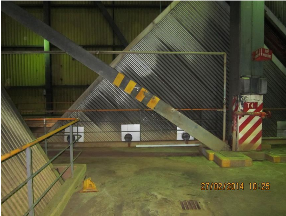
Figure 12- Unit 2 Side of Duct showing Surrounding Items and Existing Test Ports
