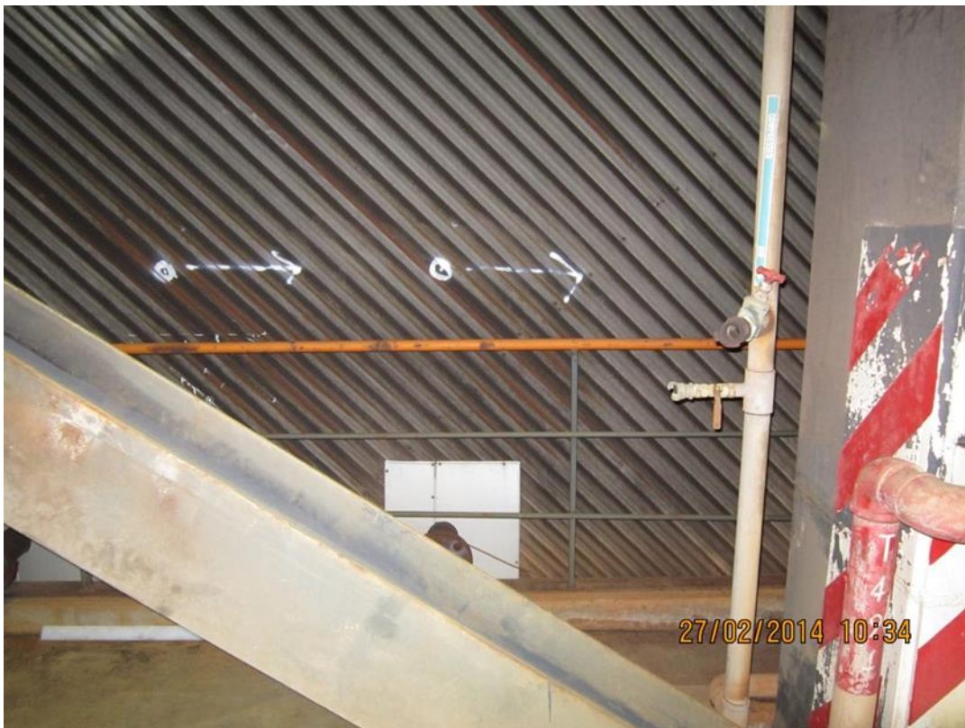
Figure 13- Preferred Location of Instruments, Turbine Side of Duct (end of arrows)
