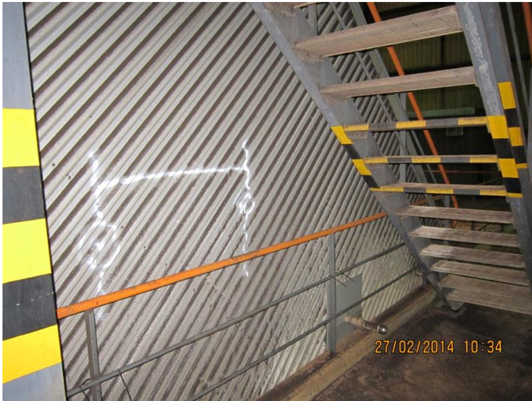
Figure 14- Preferred Location of Instruments- Precipitator Side of Duct
