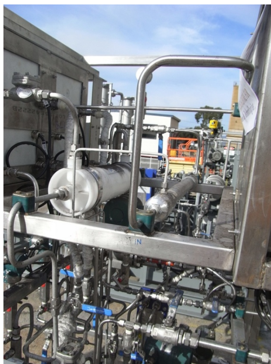
Figure 5.2.2 H3 Capture Project Membrane Pilot Plant, Gas separation membrane is on the right with the gas-solvent contactor unit on the left.
